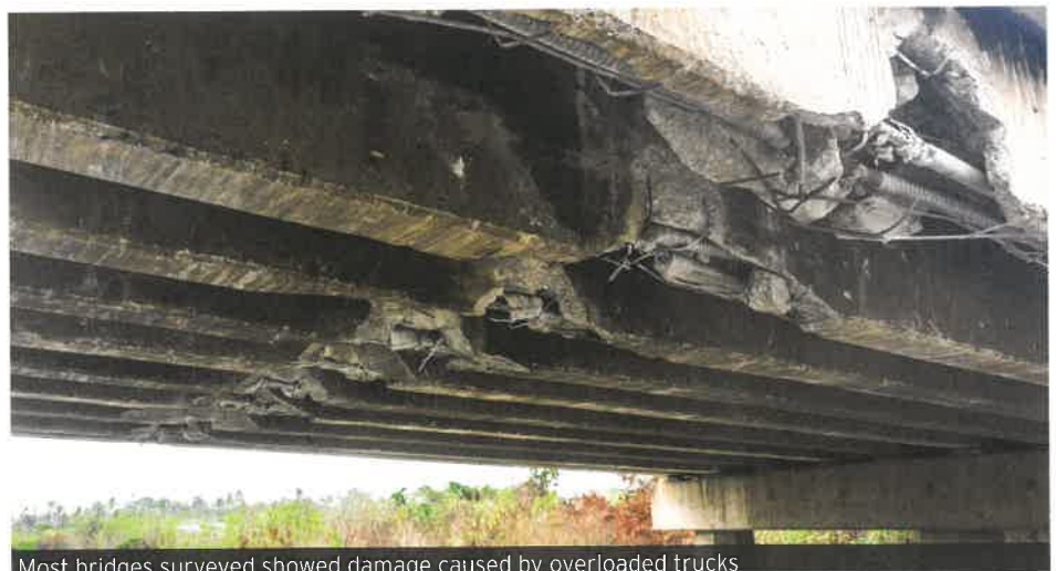
Most bridges surveyed showed damage caused by overloaded trucks
